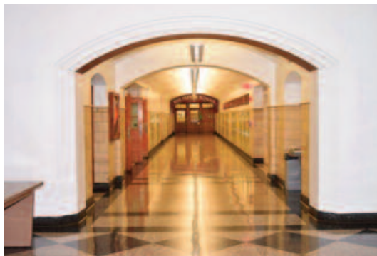
New hallway lighting
